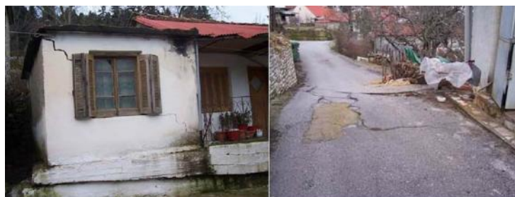
Figure 2. Kerasia village photos showing damage at houses due to landslide
